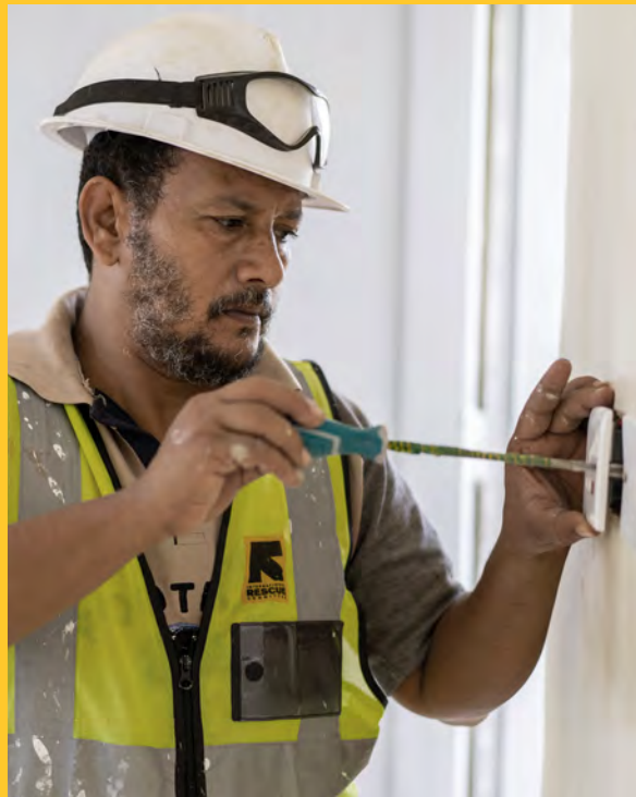
Yasser Omar, 50, attaches an electrical switch to a classroom wall in Abyan, Yemen. An IRC cash-for-work project to rehabilitate a local school has enabled Yasser, a former fisherman, to make a more sustainable income.
